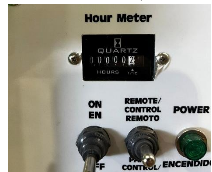
New Electrical Panel depicts 0 hours
